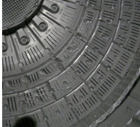
Ball Mill Discharge
